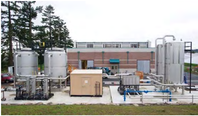
A Unison Solutions gas conditioning system is located outside of the cogeneration building.
